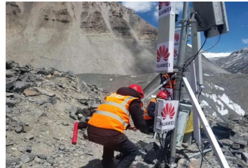
5G Site and 3 4K Cameras Installed A.S.L 5300m
